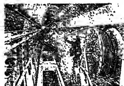
Liverpool's new 7,360 ft. tunnel under the Mersey relies on BICC cable servicing the various complex systems that ensure the smooth flow of traffic.
